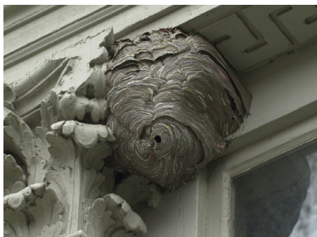
Figure 2.23 Colony of bald-faced hornets on a building.
