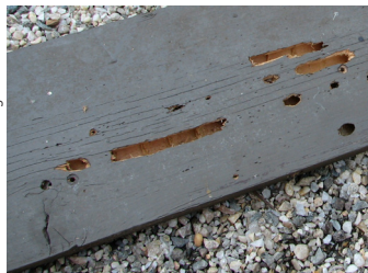
Figure 2.39 Carpenter bee galleries in structural wood.
